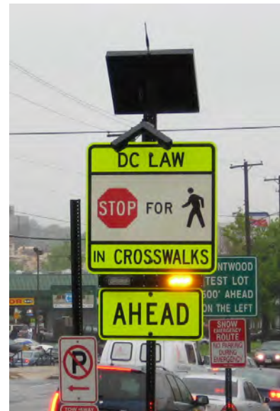
Rapid Flash Crosswalk Beacon on Brentwood Road, NE
