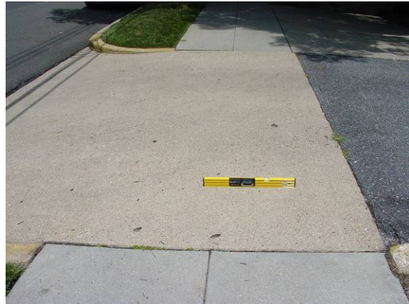
Figure 4 – ADAAG compliant driveway design at 4000 Tunlaw; 2% cross slope, full width sidewalk, and no cracks or offset joints.
