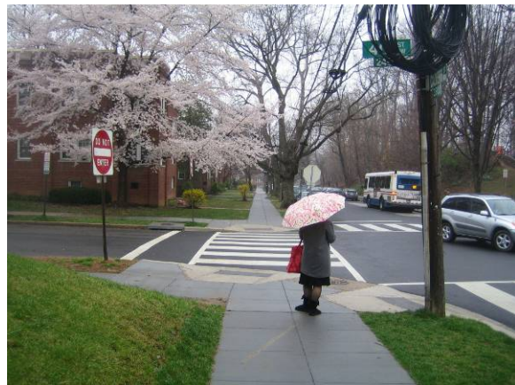
Figure 2 – Reconstructed sidewalk on Calvert at 40 th Street, restriped crosswalks, and repaved roadway
